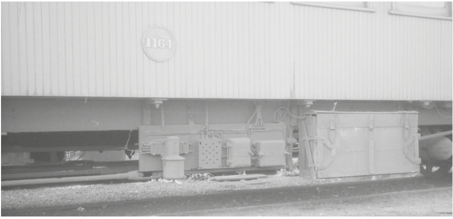
Left: Details of the electrical equipment on A 1164 showing both the switch gear and a battery box. Photographer unknown
